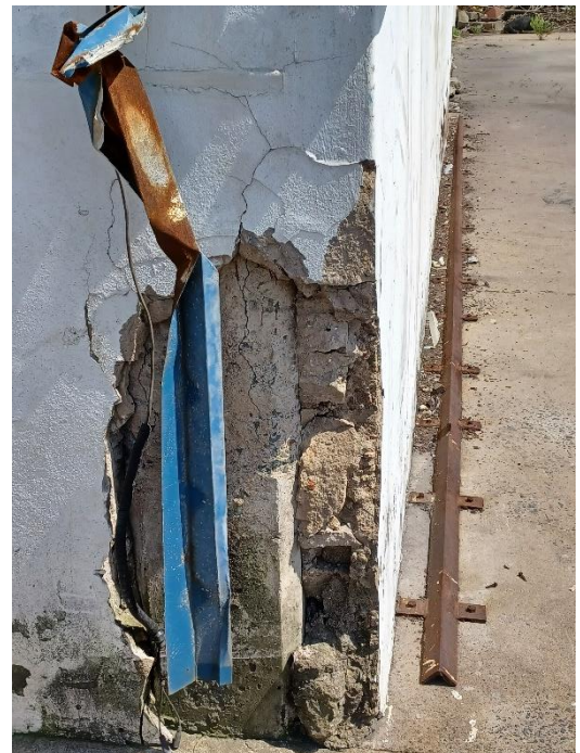
Figure 3-5: Broken brickwork/masonry at Warehouse 2.
