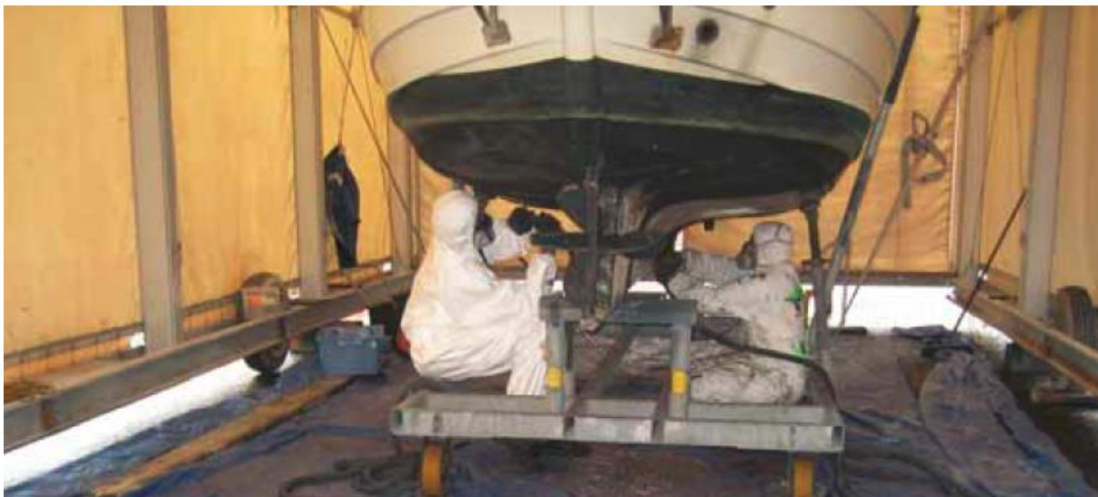
Antifouling removal and sanding done in an enclosed shed. Tarpaulin on the floor is used to contain droppings and spilled materials.
