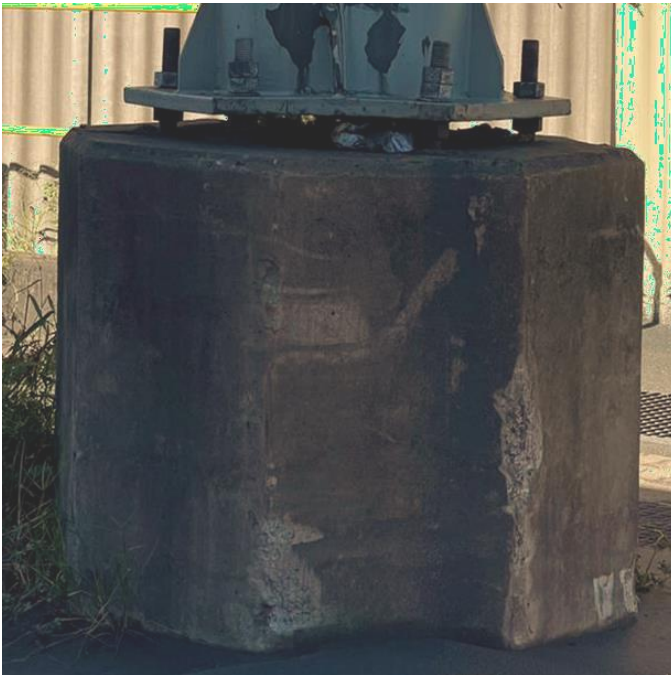
Figure 3: Spalled and damaged concrete.
