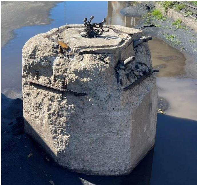
Figure 1 : Spalling, exposed reinforcement.
