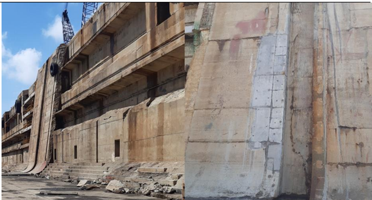
Figure 6: Spalled Concrete and Repairs to Dock Gate Groove
