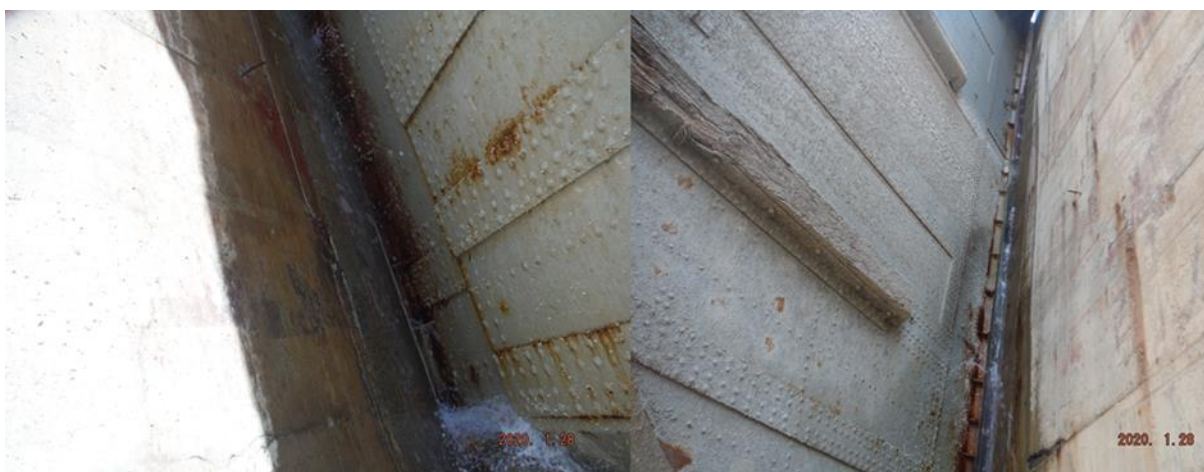
Figure 7: Leaks at Dock Gate Grooves
